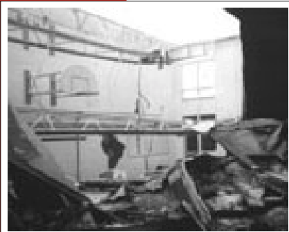
Roof fails from wet snow overload at Claypit Elementary School in Wayland, MA, 2003.
